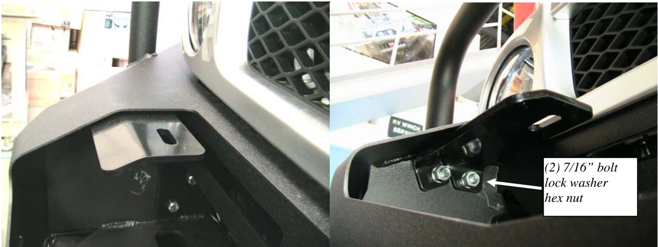
Figure 20 RH Light Bracket installed
