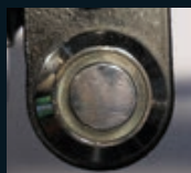
LED loop OFF valve closed
