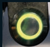
LED loop YELLOW valve 40% open
