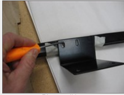
Picture #14: Align latch bracket with tape lines as a guide and scribe latch bracket holes onto grille support.
