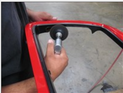
Picture #22: Use a grinder to clean up the cut area as shown.
