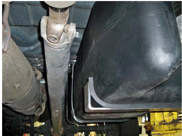
(Fig. 15) Installation of front support on tank without TITAN Shield. Note the rubber bushings on the support and the straps.
