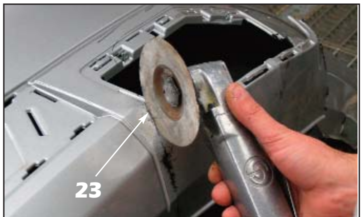
23. Using a vibrating saw or a jig saw, cut through the bumper cover on the grease pencil marks. 24. Cut the top edge flush with the upper edge of the lower recess (not shown).
