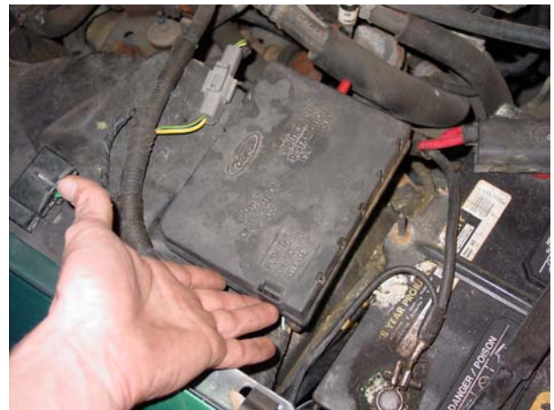
16. Open fuse box.
